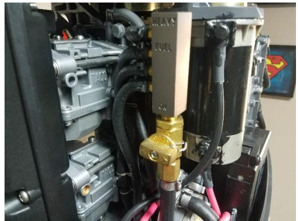
Fig (8) Raider 50HP with USCG compliant lines installed
